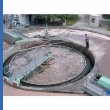
Effluent Treatment Services
