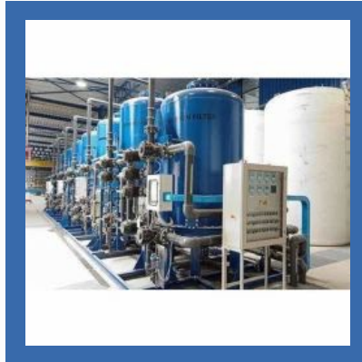
Water Demineralization Plant
