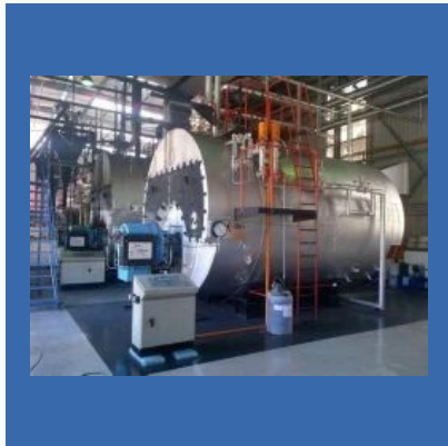
Fireside Treatment Chemicals
